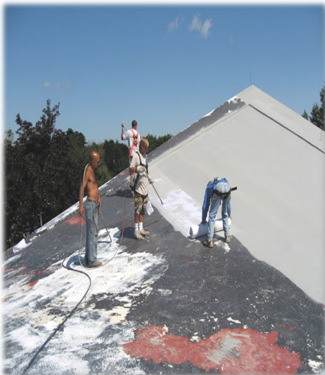
A thorough power washing revealed multiple layers of failed waterproofing attempts
