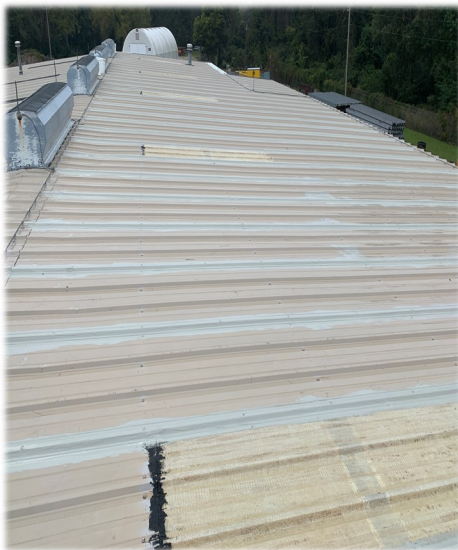
Fiberglass skylights are hard to see and create a dangerous hazard on roofs
