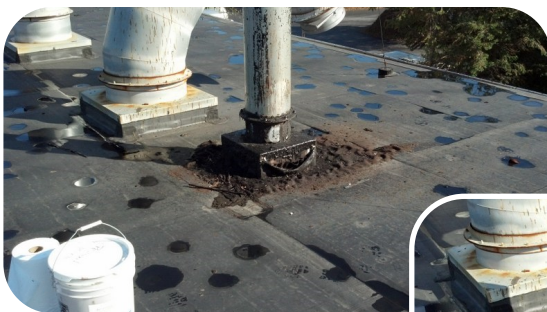
Heat destroyed EPDM Roof
