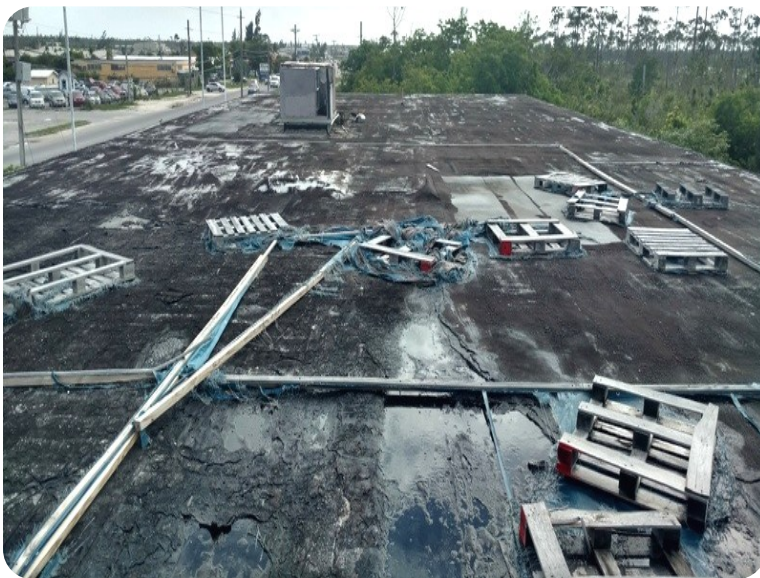
After the debris was removed from the roof, a high pressure washing was done
