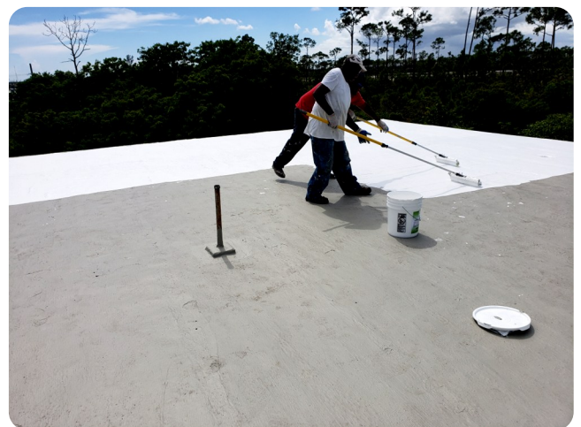
After the pressure washing and preparing the surface the Acrylabs System was installed
